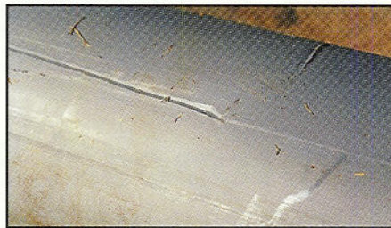
Gouge in HDPE pipe prior to insertion
