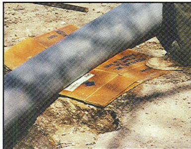
Rudimentary protection against pipe damage during installation
