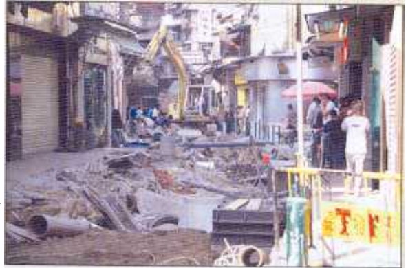
To dig or not to dig: open-cut in Macao (above) vs. HDD in Amsterdam.
