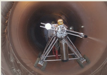
Fig 13. A robotic unit used to apply a 60 mil polyurea coating to nearly half a mile of 96" and 72" steel pipe.
