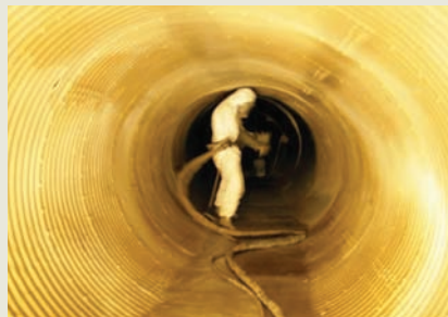
Fig 14. Application of a 250 mil of polyurethane coating for the rehabilitation of a 60" CMP culvert.
